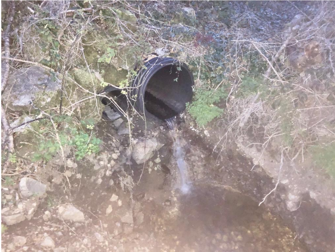
Plate 2-1 View of 600mm N59 road culvert for the Glenlo stream (this section is likely to be an extension and possibly an older stone culvert is present in the middle / upstream section of the road)
